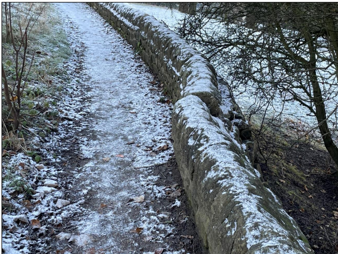
Photo 4. Damaged retaining wall north of A660 (Area 16C).
