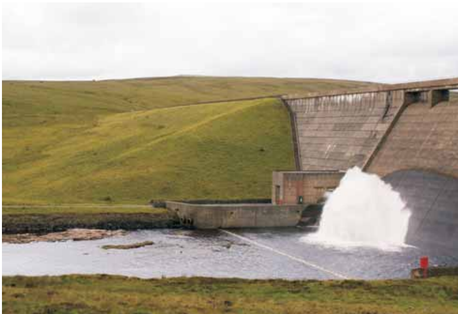
Cow Green dam wall showing the two parts: the concrete wall and the earth bank.
